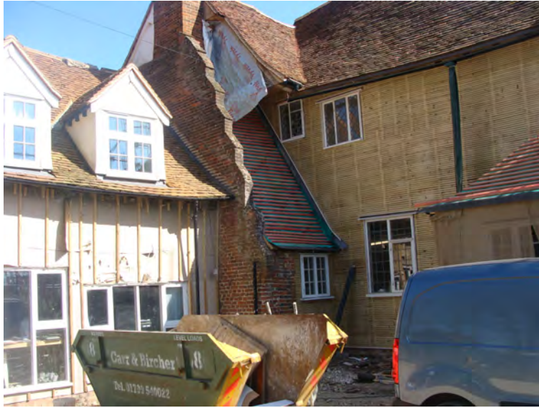
Picture 1.6 Widdington Hall, a 15th century moated hall house, currently being renovated
