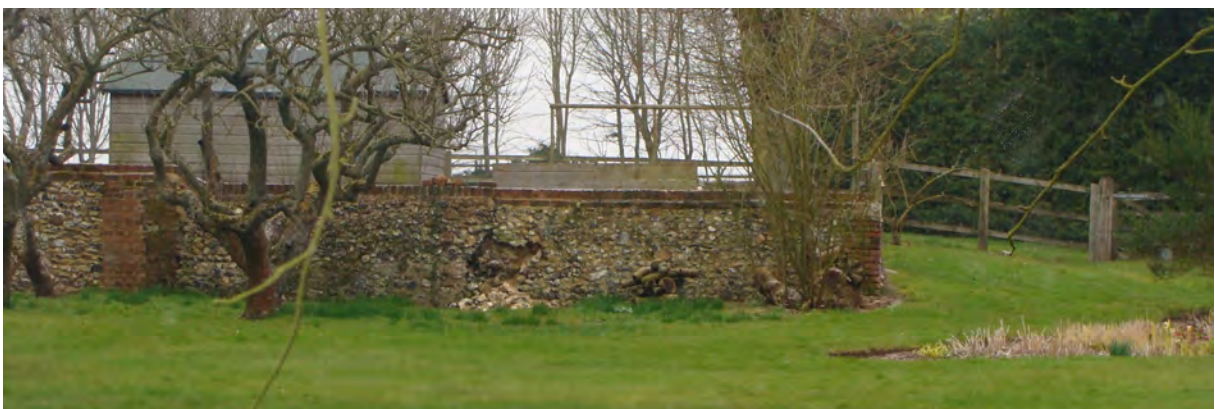
Picture 1.16 Wall at Widdington Hall in urgent need of repair
