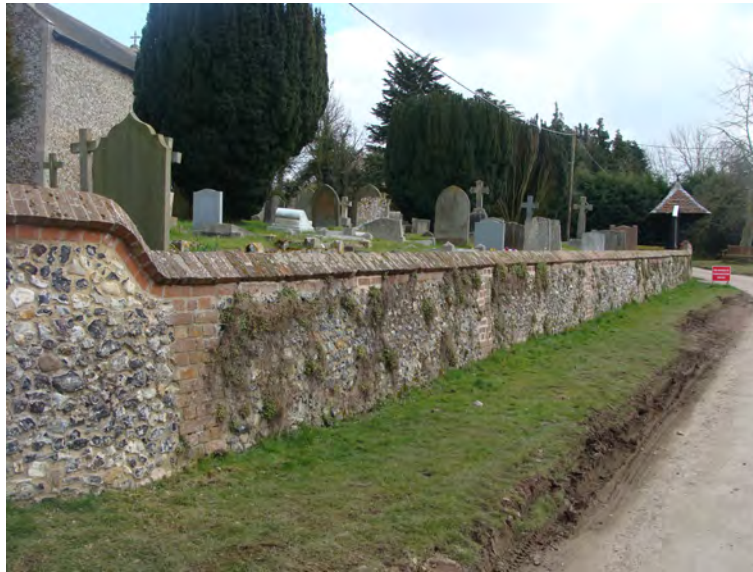
Picture 1.15 Fine boundary wall to churchyard. Acts as an extension to adjacent boundary wall to Rectory which in combination creates an environmental feature of considerable importance
