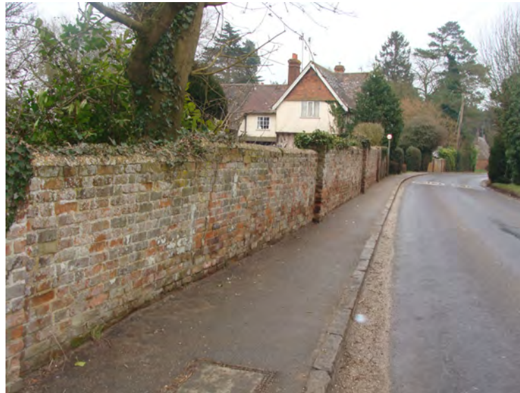
Picture 1.23 Wall fronting Pond Mead in need of some repair works and important in the street scene
